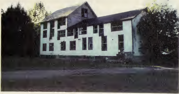
Fig. 61 Photograph of the Anselma Station depot. •The structure formerly housed a local store, a freight storage room, offices for the railroad employees, and a waiting area for passengers. It is now empty. Photograph by the author, 1994.
